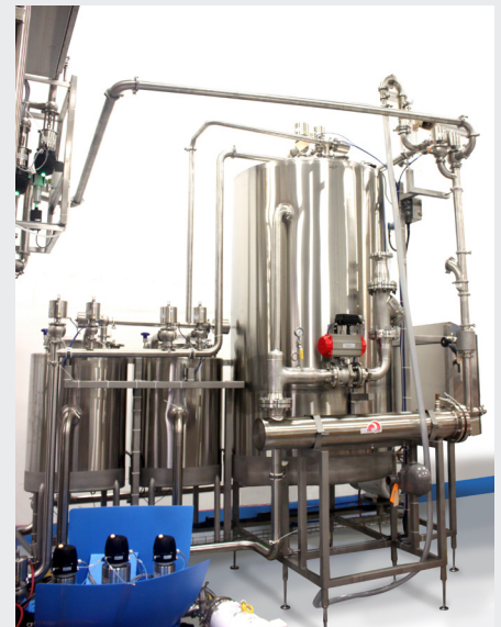
CIP Cleaning Skid
